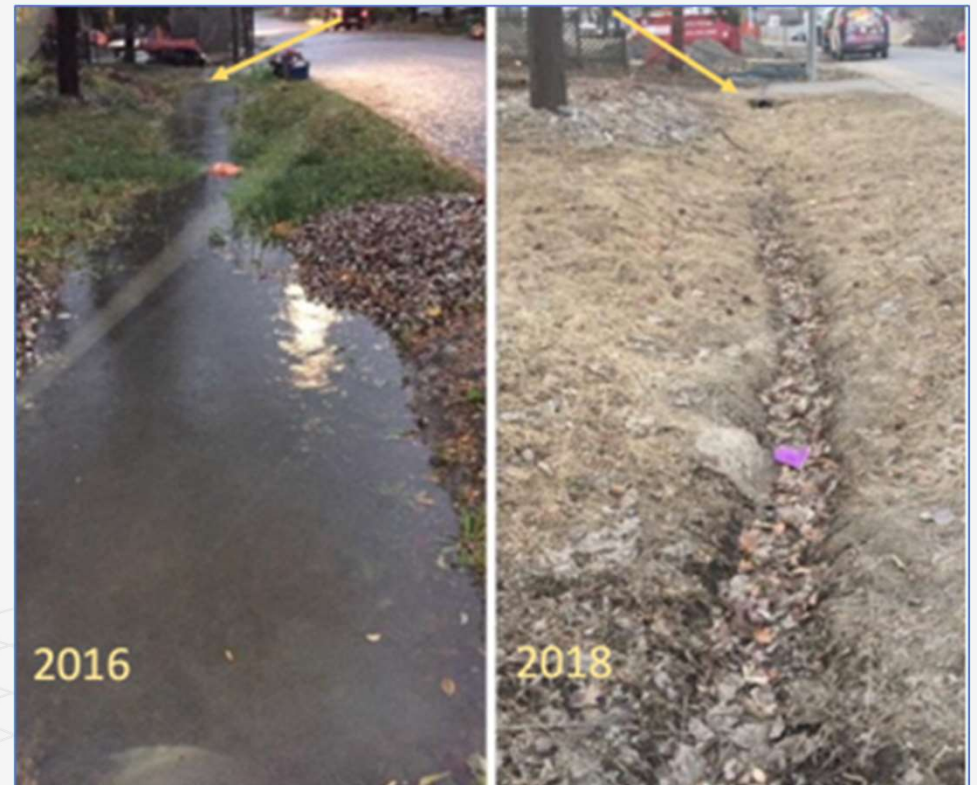
New development leaves upstream homes without positive drainage and standing water in Carleton Heights in 2016.
