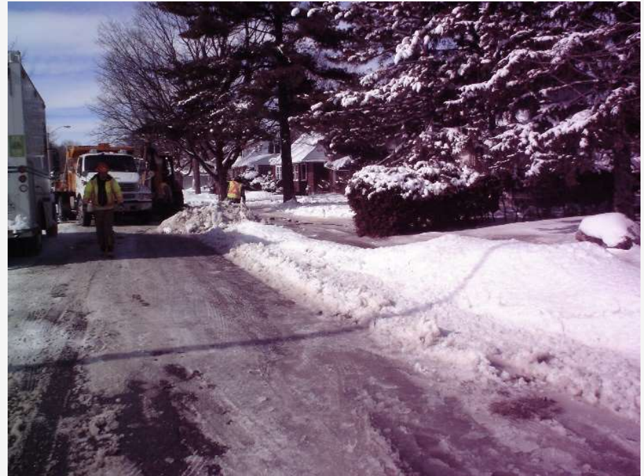
Water main needs repair in Carleton Heights (2020)
